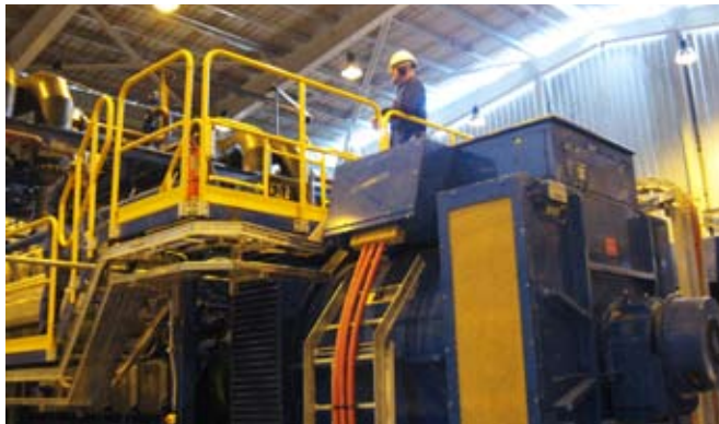
Natural gas-fired Wartsila units are the primary power generating devices at Piriquitas.
